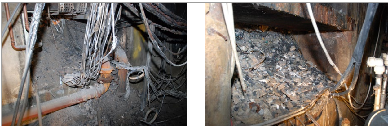
Figure 19 – Cables exiting vertical ducts into level 2 Plenum
