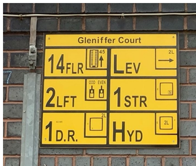
Figure 3: High rise external indicator plate in place Source: HMFSI
