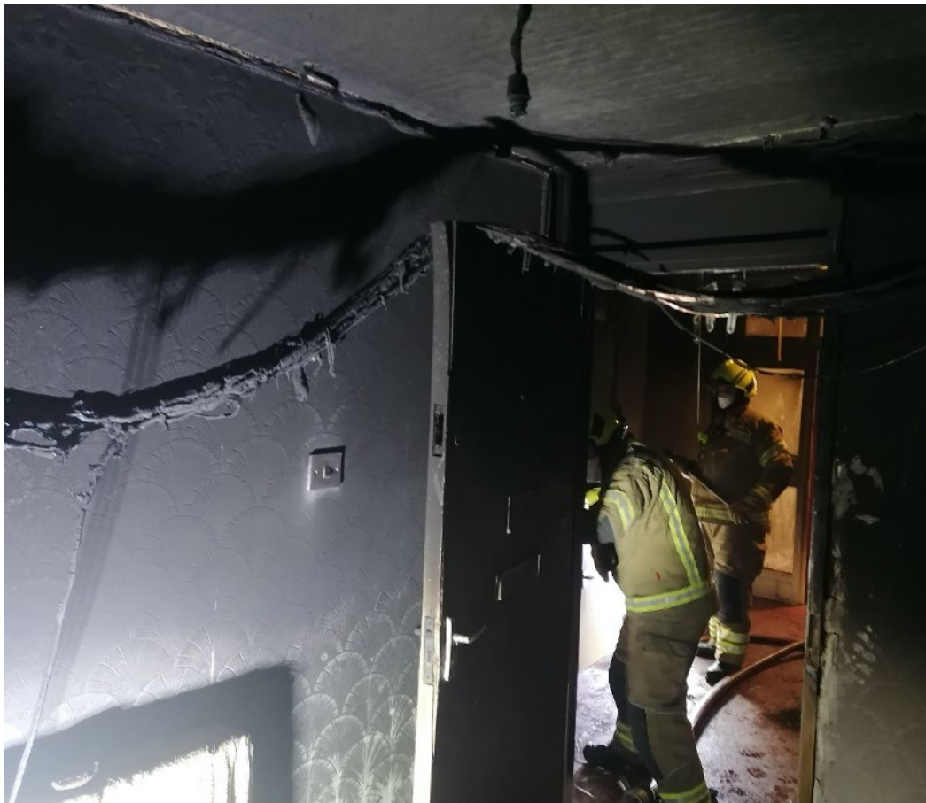
Figure 7: Dislodged cabling Source: SFRS
