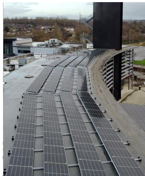
Solar Panels at SFRS HQ (Cambslang)
