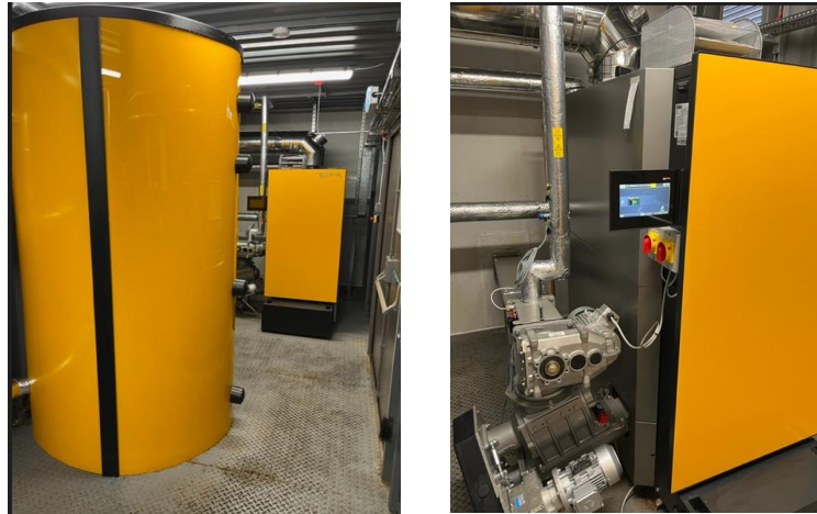
Biomass Boiler at Fort William Fire Station
